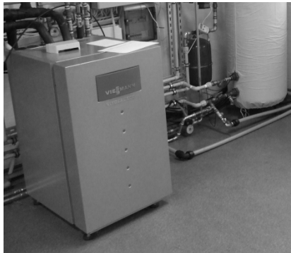
Fig. 1. The heat pump in the „Ecobuilding”
